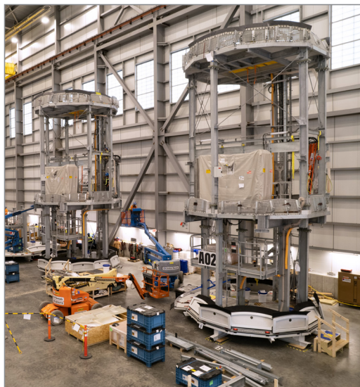
Two of twelve Supported Internal Platforms (SIPs) being constructed at our facility in ProvPort, RI for the South Fork Wind Farm.
