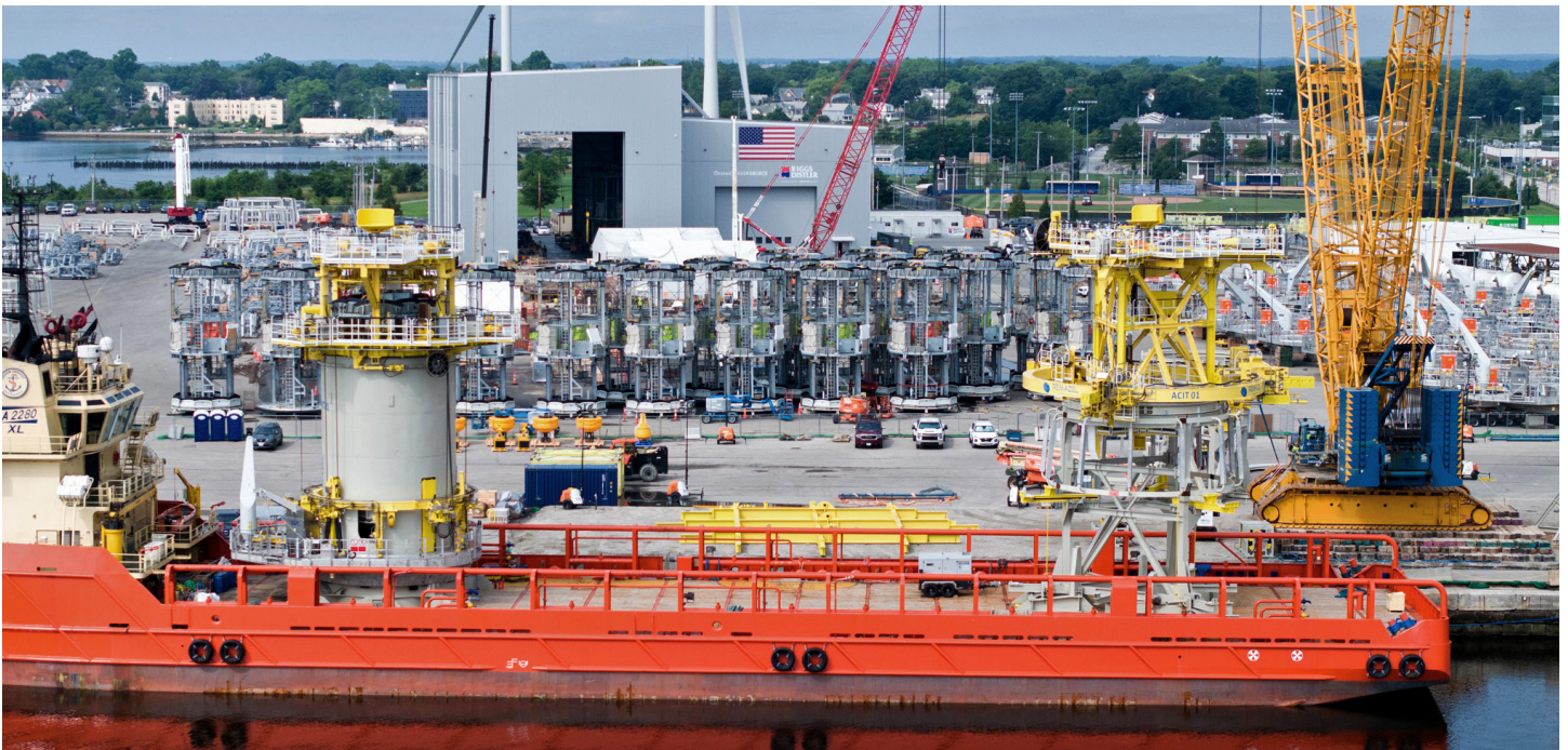
A view of the quay side of the offshore wind facility in ProvPort, RI where we are construction advanced foundation components for Revolution Wind.
